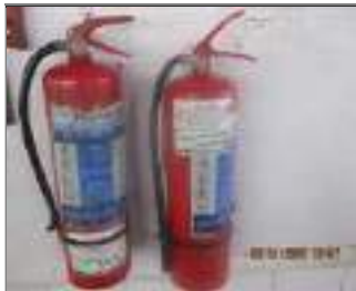
Photo of fire safety equipment Fire extinguisher.JPG
