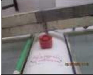
Photo of fire safety equipment Fire alarm.JPG
