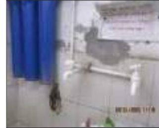
Photo of the inside of the main production hall Drinking water point.JPG
