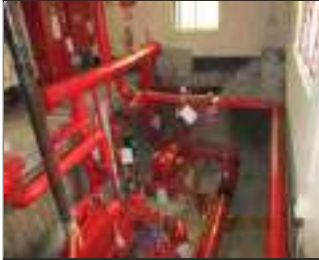
Photo of fire safety equipment Fire pump house.JPG
