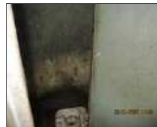
Photo of non-conformity Toilet area was found unhygienic.JPG
